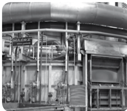
Rotary table furnace
