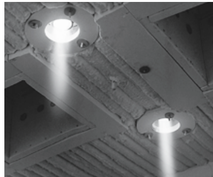
Overhead firing with burner BIC
